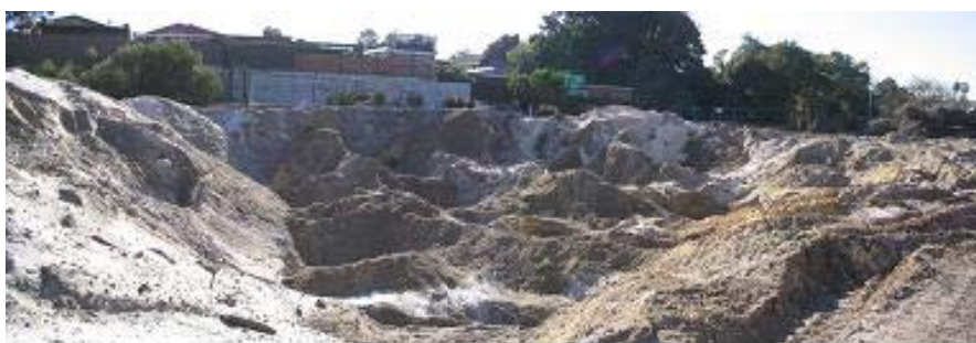
Figure 2. View of site facing north, showing former tank farm excavation prior to backfilling. (Note the proximity of existing residences.)
