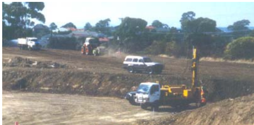
Figure 7. Field testing over the refuse fill prior to impact rolling. Impact rolling in progress on peripheral fill.
