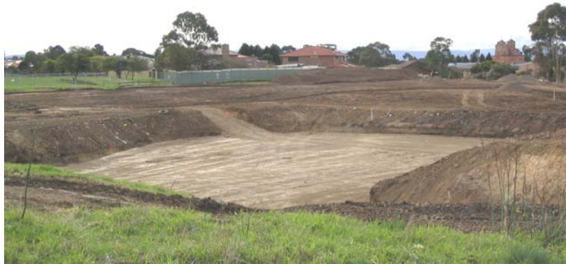
Figure 3. After excavation of the former capping over the refuse, prior to impact rolling.
