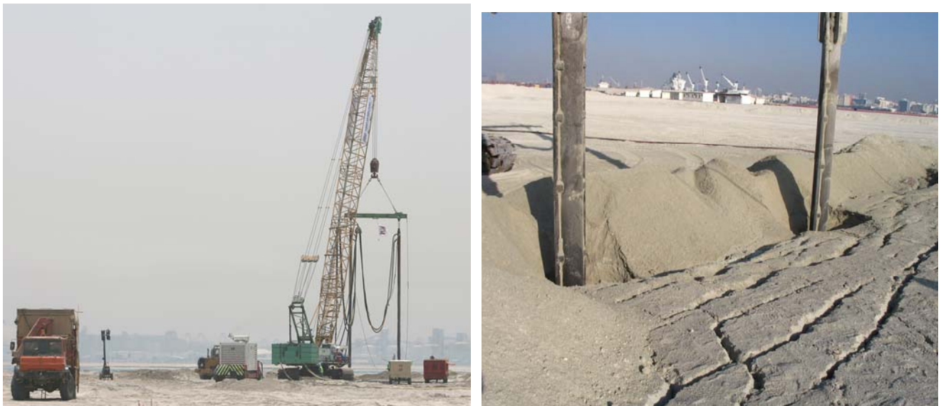
Figure 4: Vibro-compaction at Dubai Maritime City, Dubai – note craters and tension cracks.
